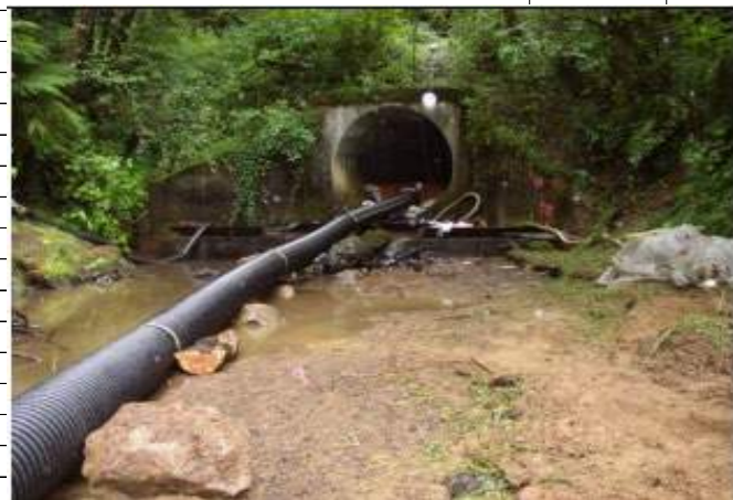
Example picture of a bypass
